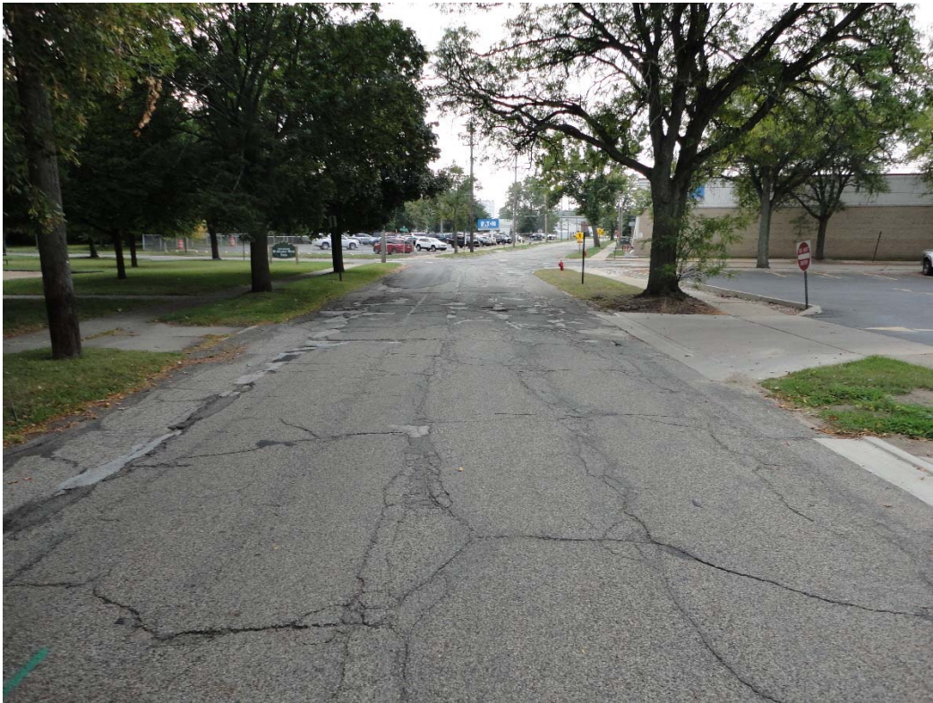
Photo 1: East Avenue in front of 200 S. East Ave looking south to Plymouth
