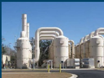
Orange County, FL Eastern Water Supply Facility (Expansion to 62.5 MGD, $26M)
