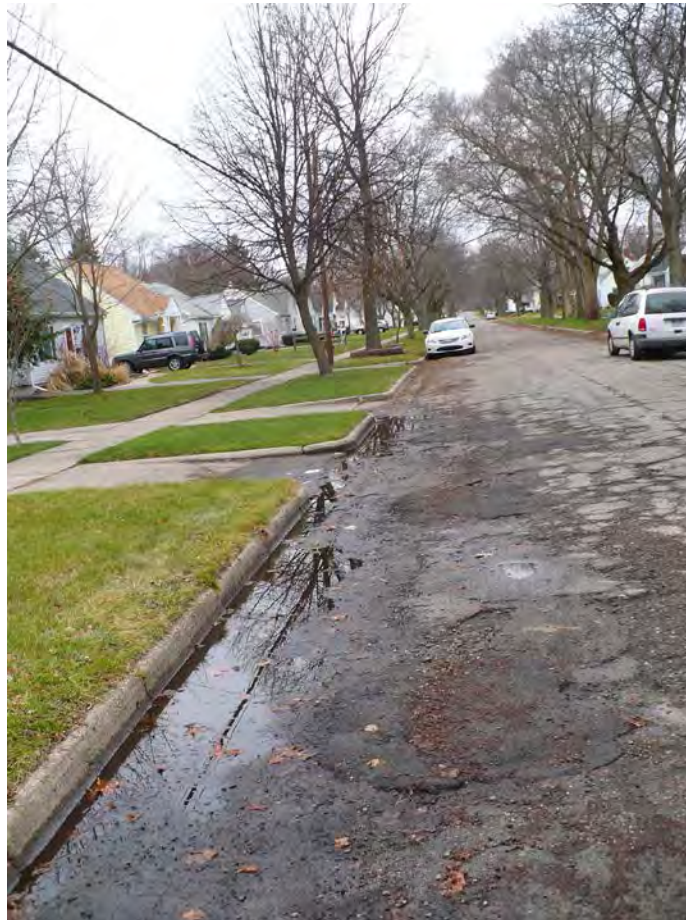
Photo 2: Curb west side facing north from Oakdale
