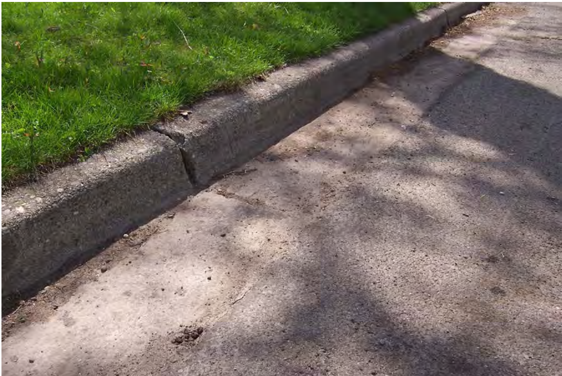
Photo 4: Typical Curb in Fair Condition
