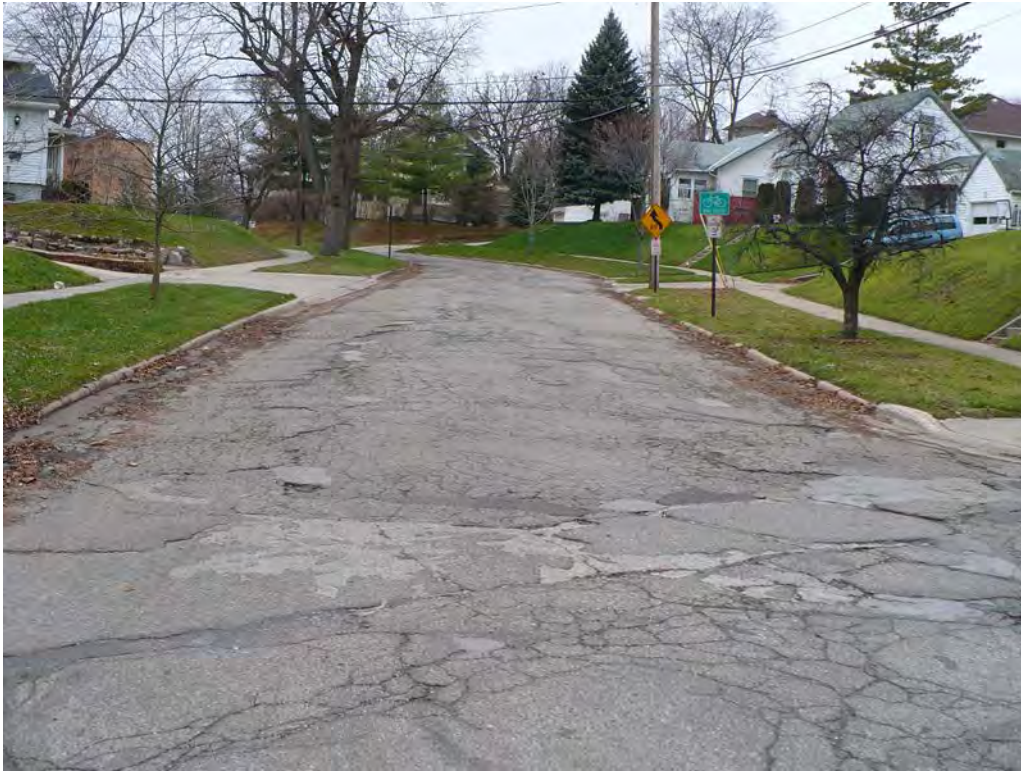
Photo 1: Condition of existing pavement facing west on Homewild Avenue from Edgewood Street
