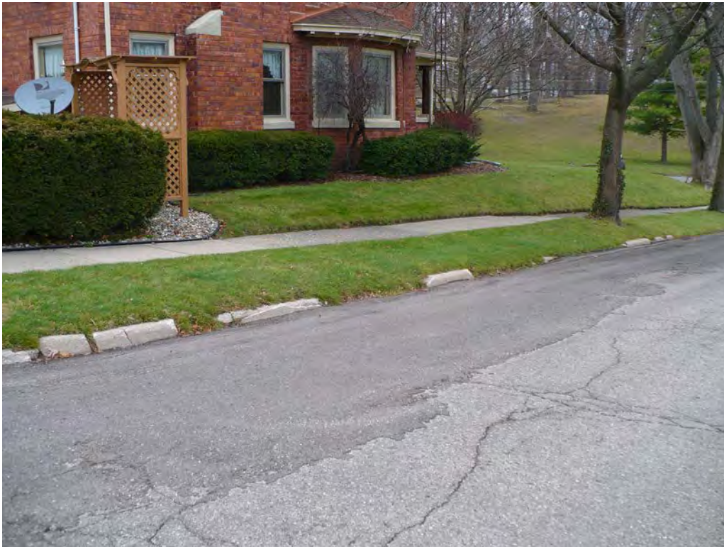
Photo 6: Condition of existing curb and gutter on north side of Forest Avenue west of Edgewood Street
