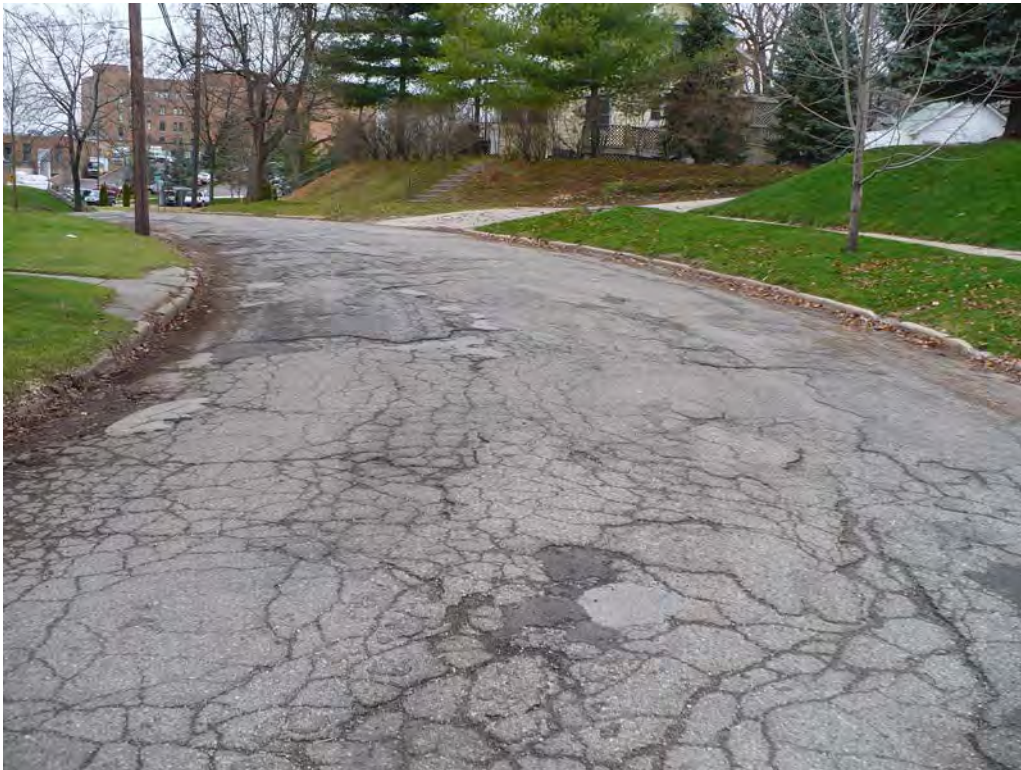
Photo 2: Condition of existing pavement facing west on Homewild Avenue from mid-block
