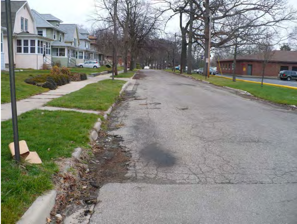
Photo 3: Condition of existing pavement facing east on Forest Avenue from west bend
