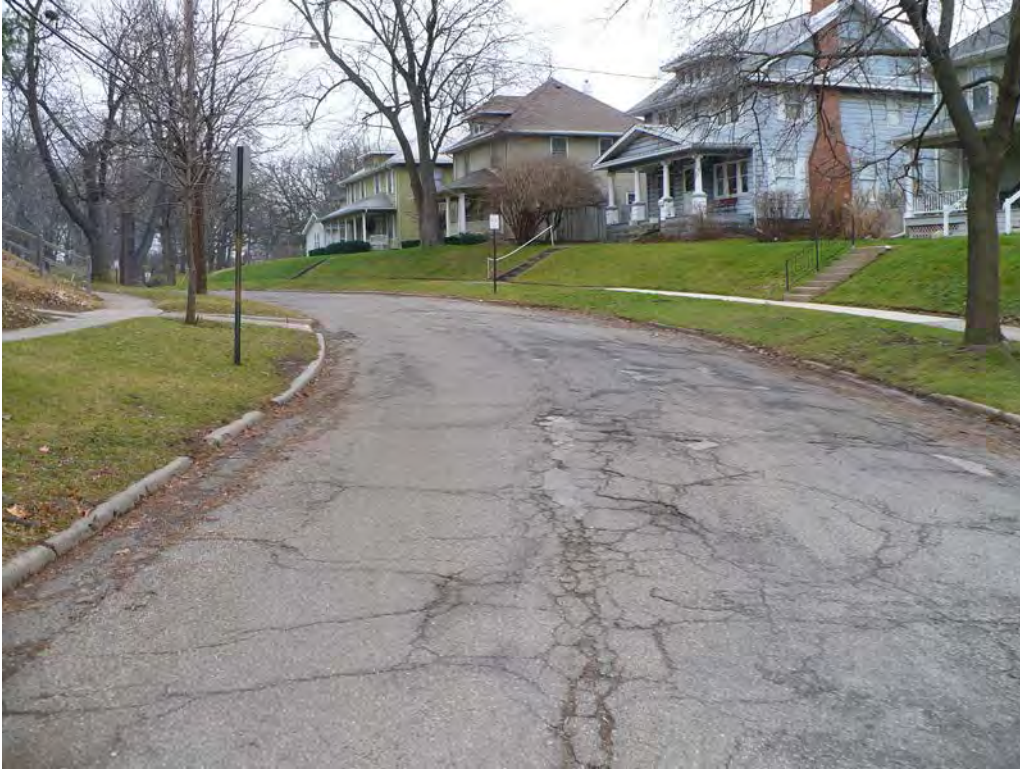
Photo 3: Condition of existing pavement facing east on Homewild Avenue from Ellery
