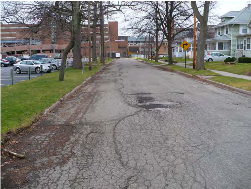
Photo 2: Condition of existing pavement facing west on Forest Avenue from mid-block
