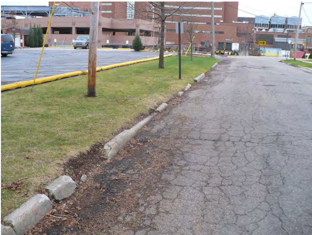
Photo 4: Condition of existing curb and gutter on south side of Forest Avenue at mid-block between west bend and Edgewood
